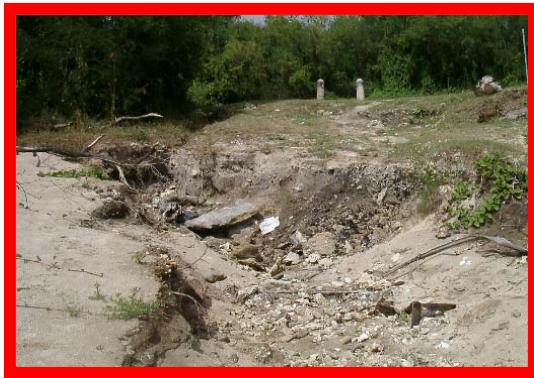
Erosion at base of access road.
